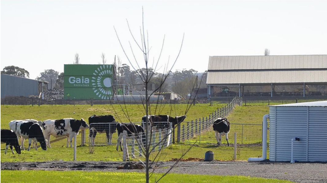
Gaia EnviroTech Biodigester installed at a Victorian dairy operation
